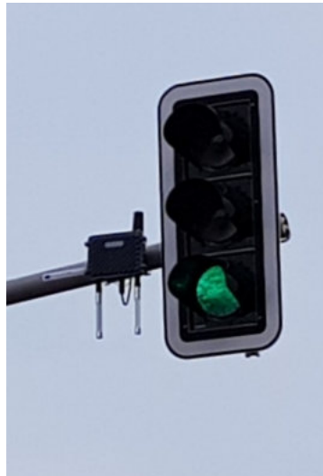
Figure 69 - R-ITS-S at traffic light
